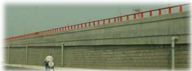
Fig. 19: Drain Pipe without any cover
