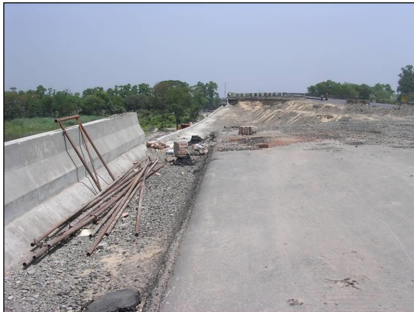
Photo 6 and 7: Case of Deep Seated Failure
