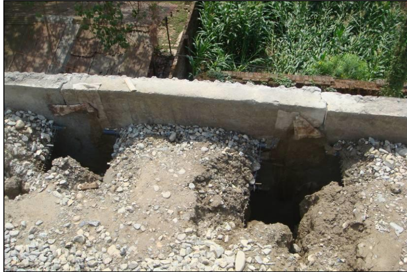
Photo 5: Case of Sand Loss Due to Rainwater
